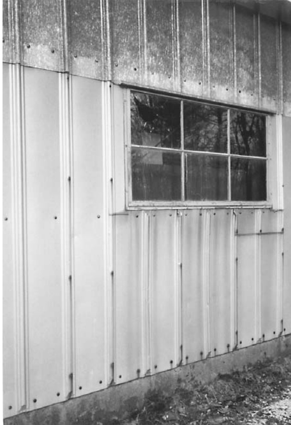
FIGURE 7.11 Rusted screws in through-fastened wall panels.
